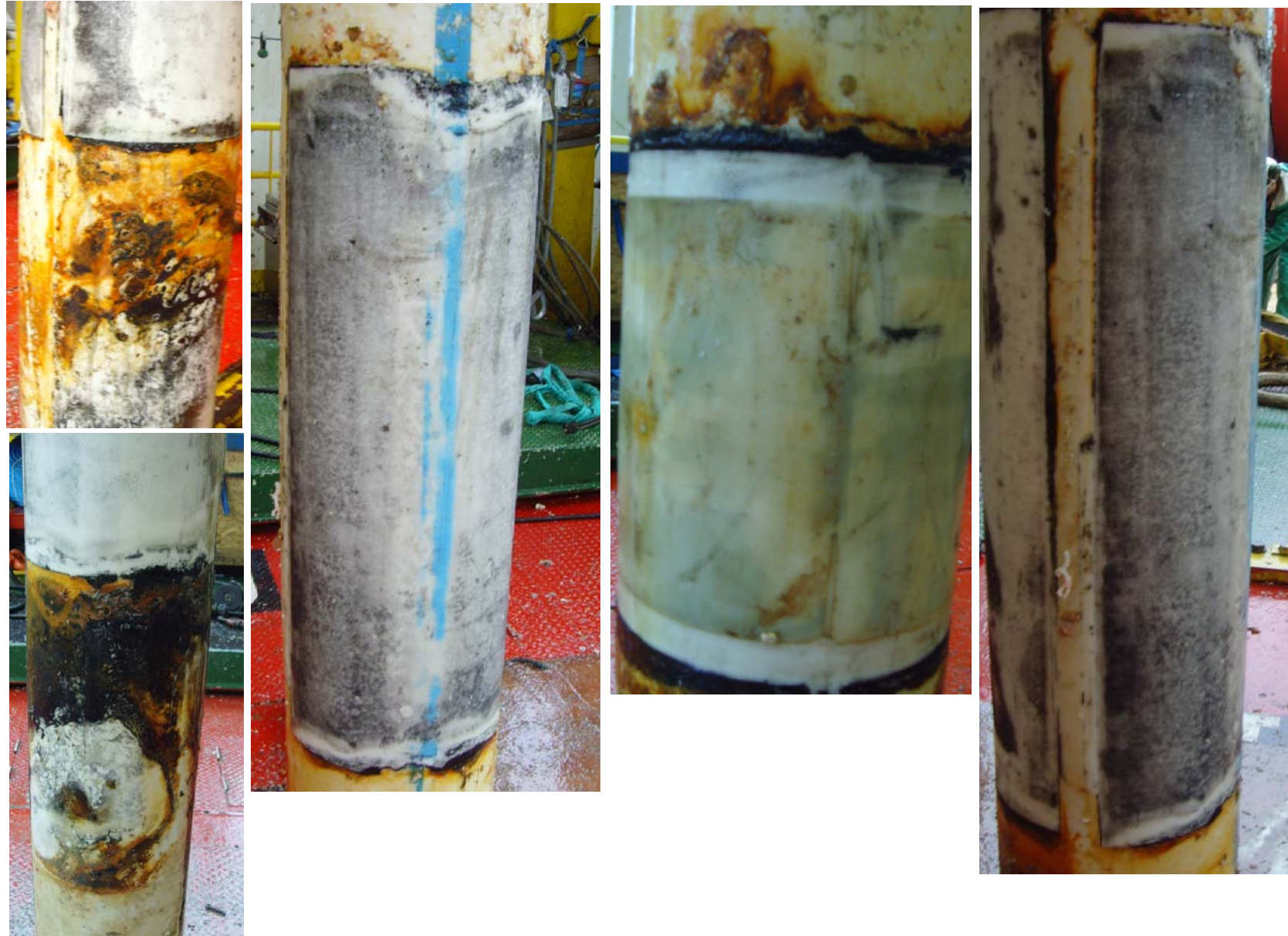
External sheath condition under repair clamps / tether clamps and adjacent to rigging
